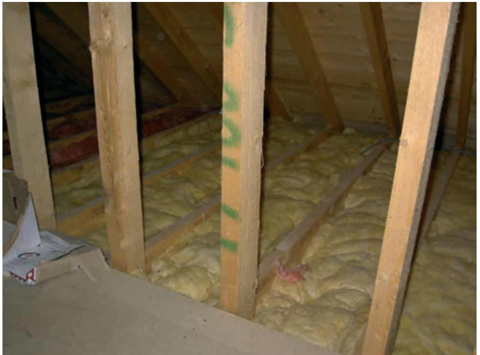
A loft like this one at Spey Bay Hall can top up the roll-out insulation to make it up to 275-300mm
